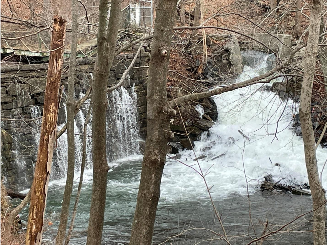
Figure 9: Heavy water flow from spillway and leaks in dam visible at time of visit, facing north east (12/19/23).
